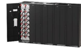
In Room Lithium-ion Battery Cabinet
