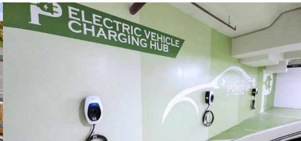
First EV Charging Solutions Certified by Philippine Safety Standard
