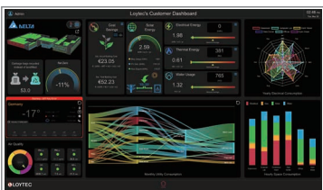
Building Management System (L-WEB)
